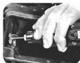
Cut off bolts
